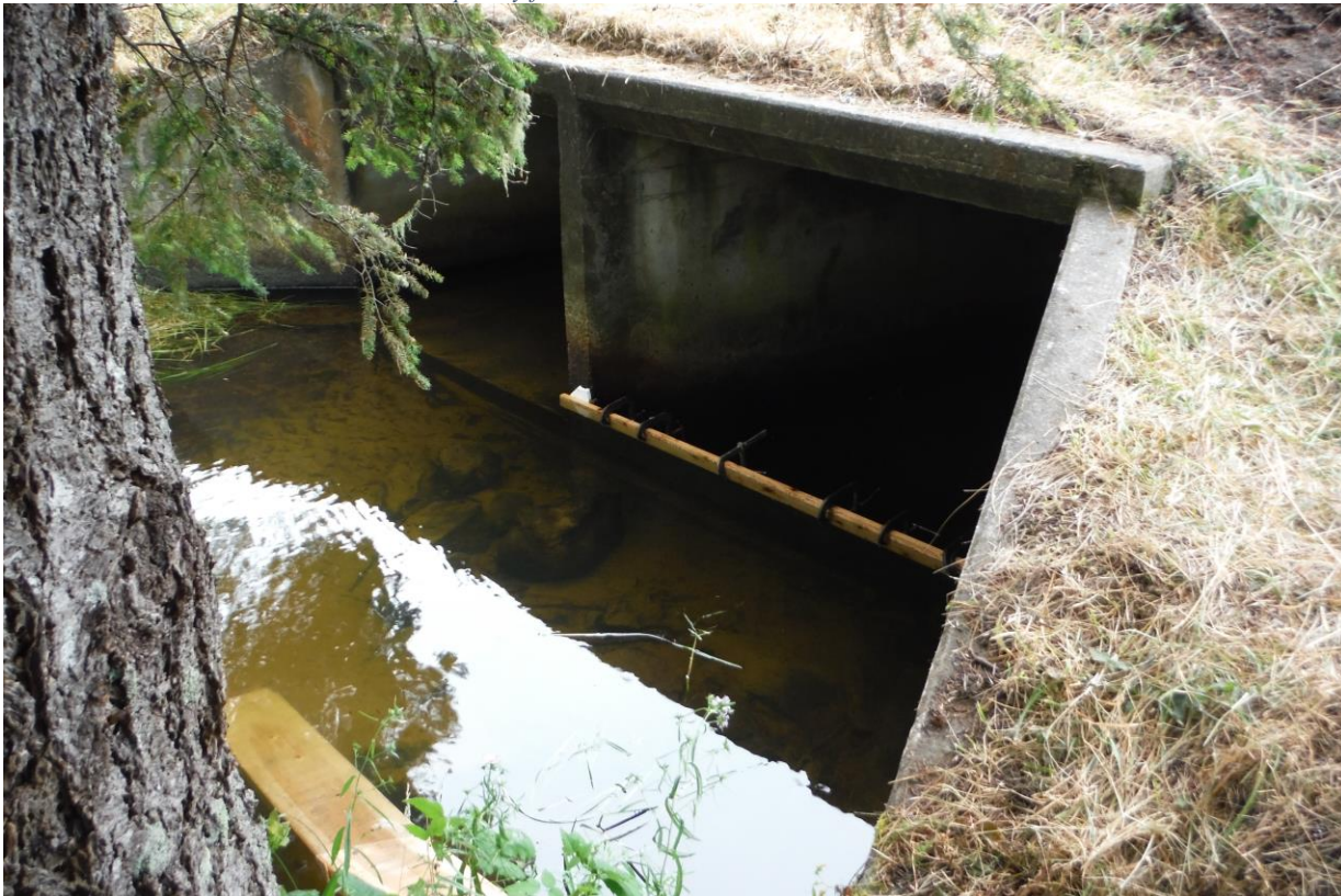
Photo 25- SC #E3 –Inlet with ODOT's temporary flow restrictor. 8-8-2017
